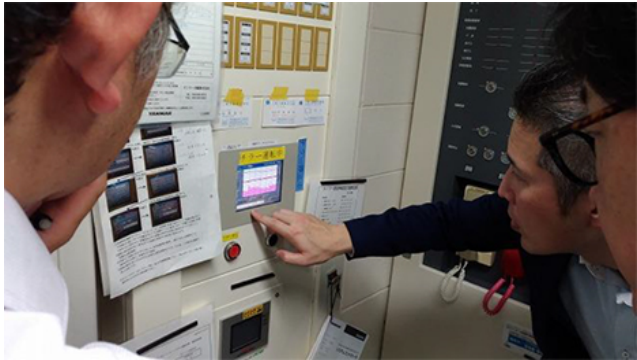
Energy consumption diagnosis at SS30
