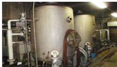
Example of reuse of wastewater: Water filtration system at Shinjuku Washington Hotel Honkan
