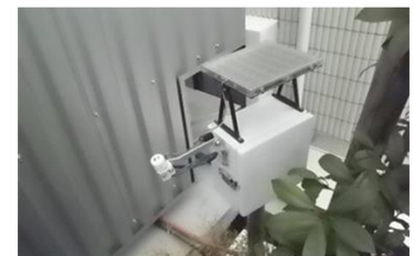
Example of water conservation equipment: Water sprinkler equipment at Luz Jiyugaoka
