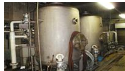
The Filtration System
